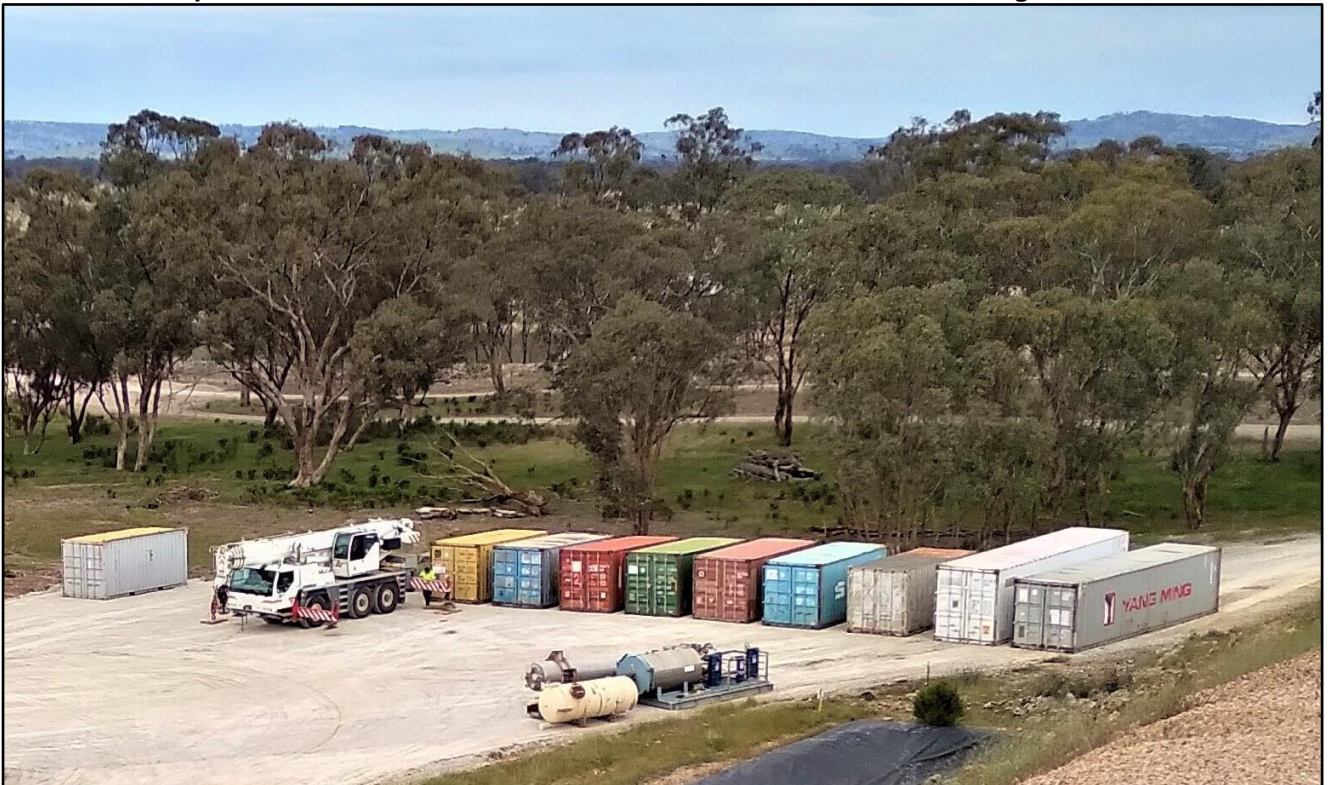
Photo 1 Components for the Gold Toll Treatment Plant in containers at the Nagambie Mine
