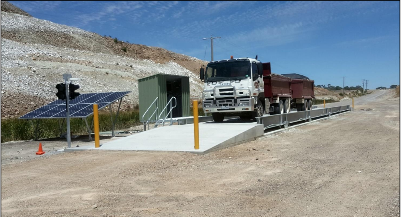
Solar panels (on the left) charge lead crystal batteries (in the green shed) that power the Accuweigh weighbridge system. The driver-controlled computer station, touchscreen and docket printer are also in the green shed.
