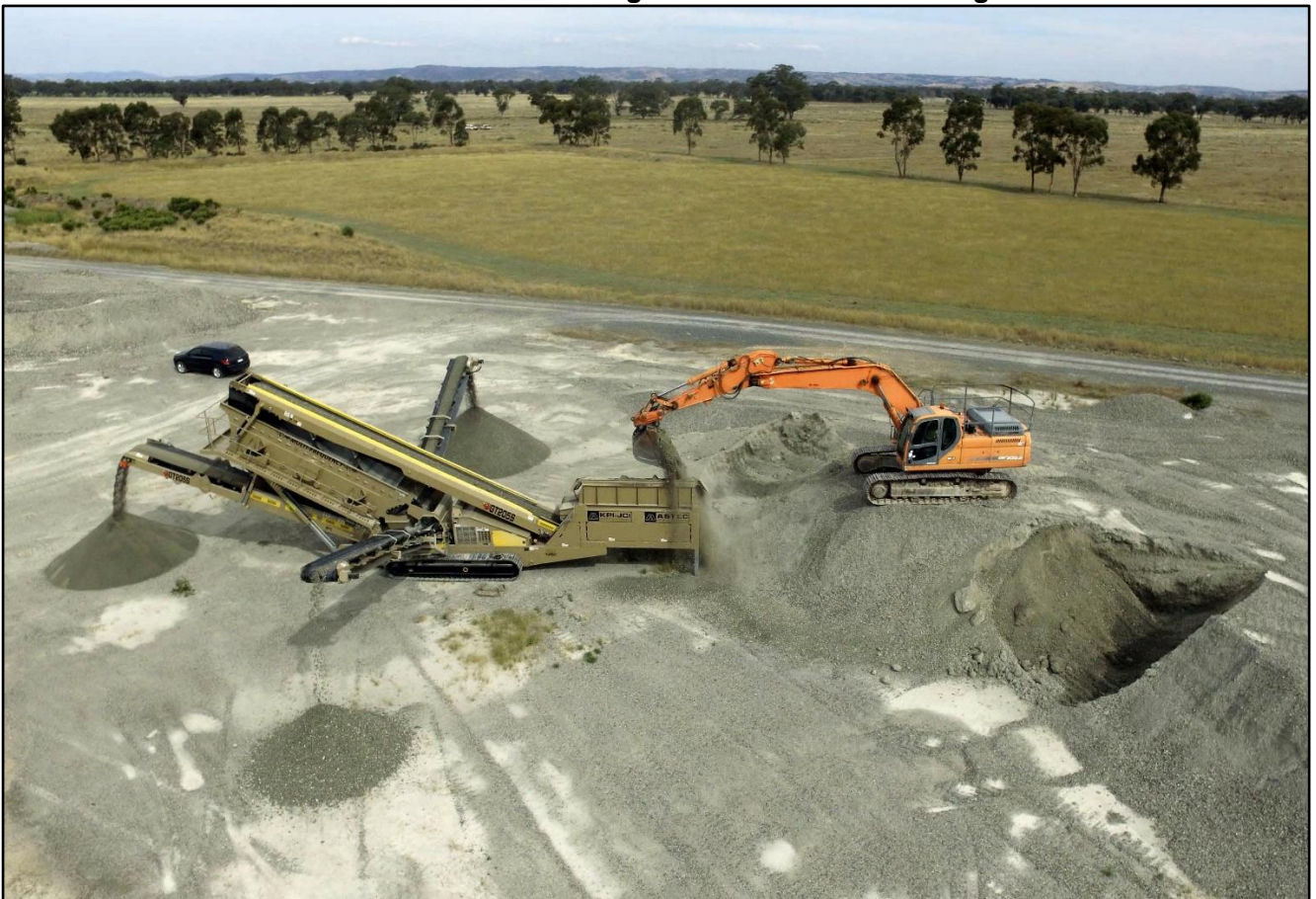
30 tonne excavator loading the hopper which has a 150mm grizzly. Product stockpiles are: Coarse (40mm aggregates), nearest to camera; Medium (20mm gravel), furthest from camera; and Fines (crusher dust), furthest from excavator.
