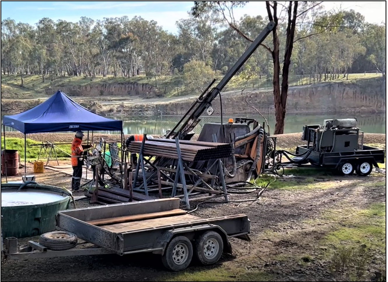
Photo 5 Diamond Drilling Rig – from this position, it drilled NAD009 & NAD010 and is drilling NAD011
