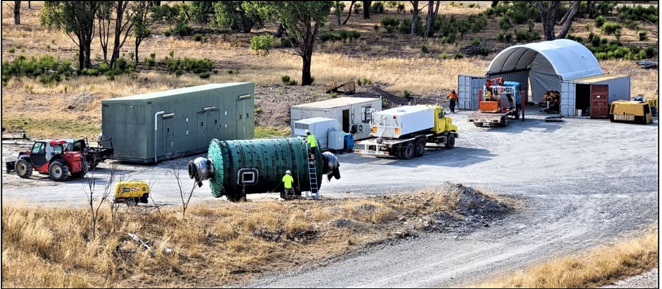
Photo 1 Refurbishment of the ANI Ball Mill (in foreground) underway for the Gold Toll Treatment Plant
