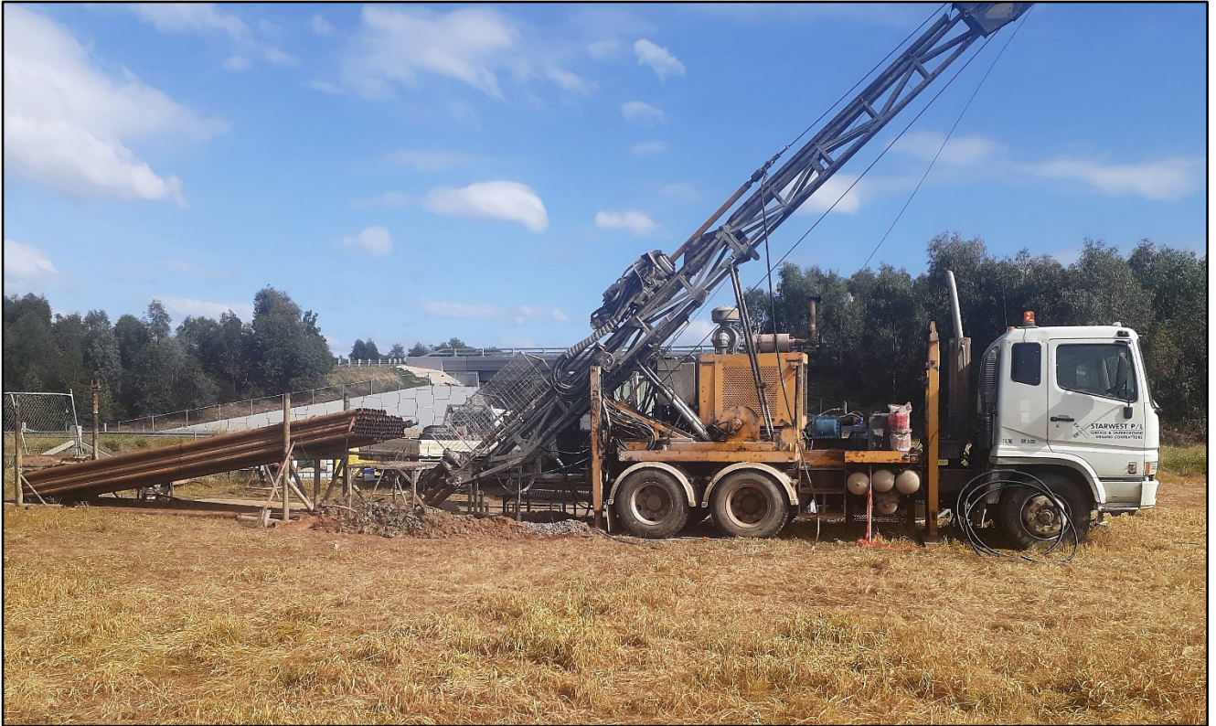
Photo 2 Looking West - RAD002 Mast 43°, Racecourse Road Underpass / Nagambie Bypass Freeway
